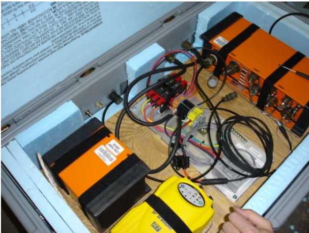
Room for geodetic GPS and seismic equipment – room for up to 600Ah battery bank under electronics.
