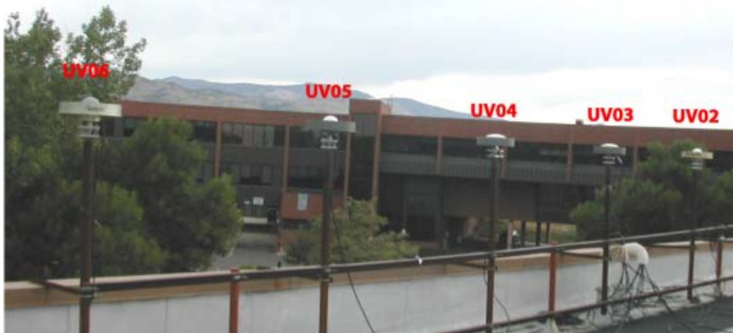
Figure 2.3- Antenna-mounting system on the roof of the UNAVCO building, looking northwest.
