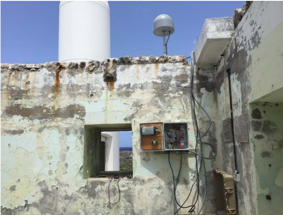
Figure 7. CN51 installed on top of the former barracks for the lighthouse staff.
